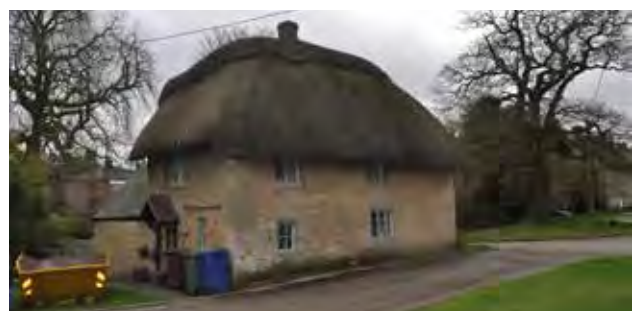
The roof form has been altered and the bay window has been removed and bricked up. The traditional flush ridge has been replaced by a block ridge which is not a traditional detail in the District.
