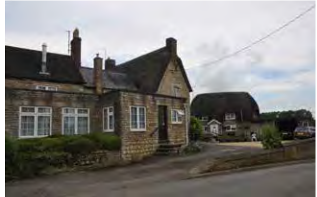
The small pitched roofed stone structure with chimney and the glazed lean-to have been replaced with an unsympathetic flat roofed extension. Flues and chimneys have also been added.
