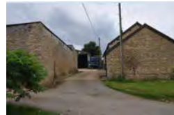
Stone Barns south of the Threshing Barn – may be curtilage listed to Old Montague House
